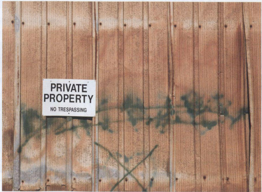
Graffiti is a common form of vandalism.
