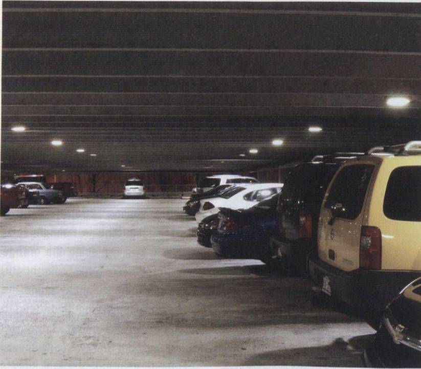
The newly installed LED lights in the City of Raleigh's, N.C., parking garage, consume 80 percent less energy than traditional bulbs and last up to 50,000 hours.
