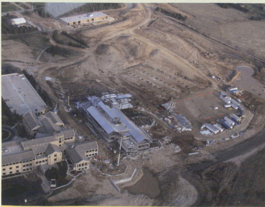
Currently under construction, West Bend Mutual Insurance's headquarters in West Bend, Wis., features an integrated system that includes climate controls, lighting, electrical and other operations systems. The security system is not integrated.
