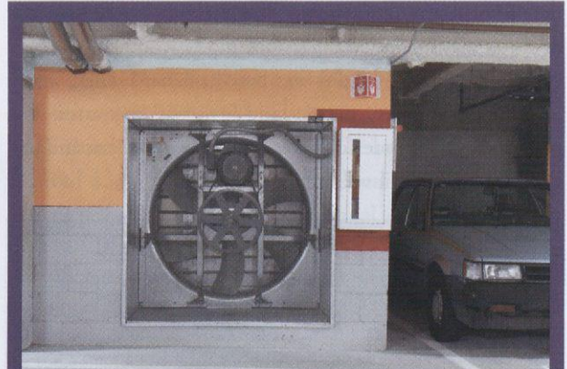
Adobe significantly reduced its energy consumption by running garage exhaust fans during high-volume periods, instead of running them constantly.
