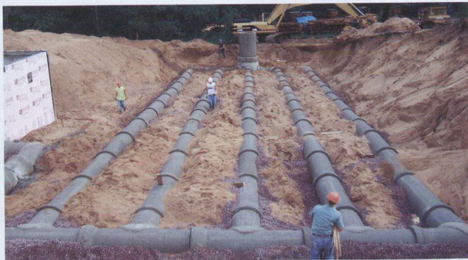
The Aldo Leopold Legacy Center reduces energy through a system of earth tubes that preheat ventilation air during winter and pre-cool air during summer.
