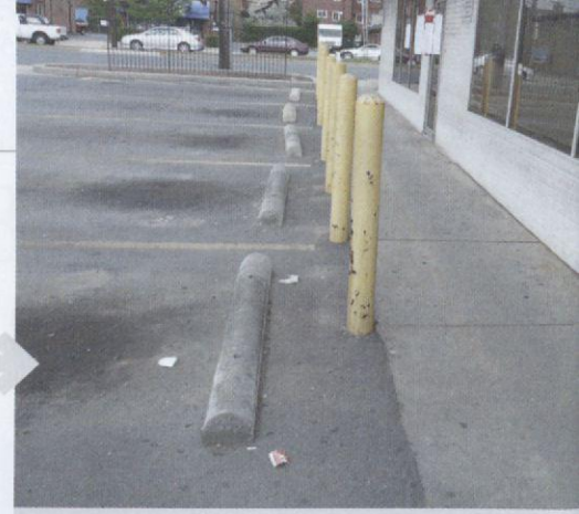
THE COMBINATION OF THE GRIME BUILDUP WITH CONTINUOUS DRIPPED OIL REPRESENTS A PEDESTRIAN SLIPPING HAZARD.
